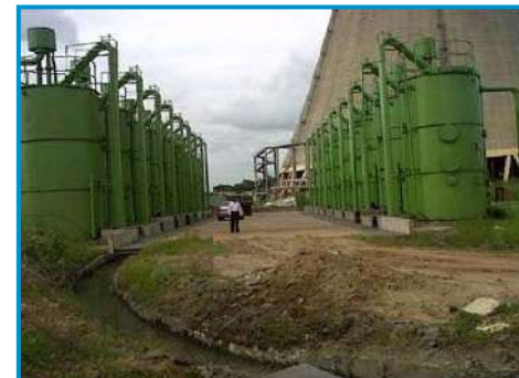
18 Nos. VAG Filter at Durgapur TPS, DVC, West Bengal thru BHEL
