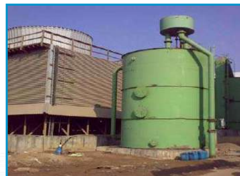
2 Nos. VAG Filter at Vedanta Jharsuguda thru HDO
