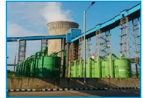
12 Nos. VAG Filter at Meija TPS, DVC, West Bengal Thru BHEL
