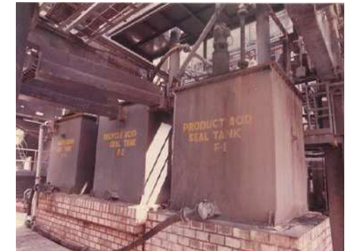
FILTRATE RECEIVER SEAL TANKS
