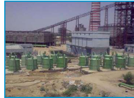
16 Nos. VAG Filter at RRVUNL, Rajasthan, thru Indure
