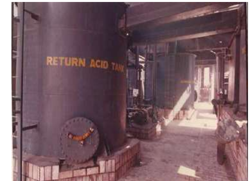
FILTRATE RECEIVER TANKS
