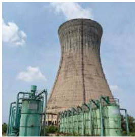
VAG for Cooling Water Treatment Plant
