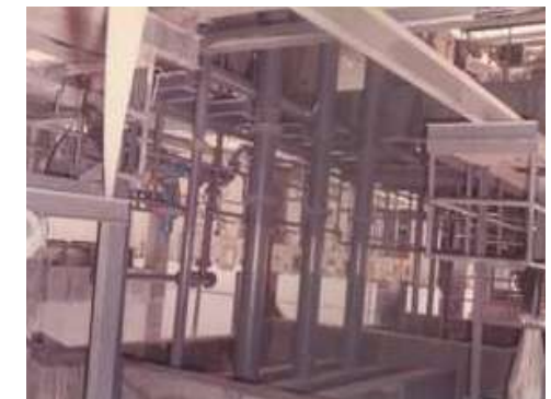
PIPING FOR FILTRATE
